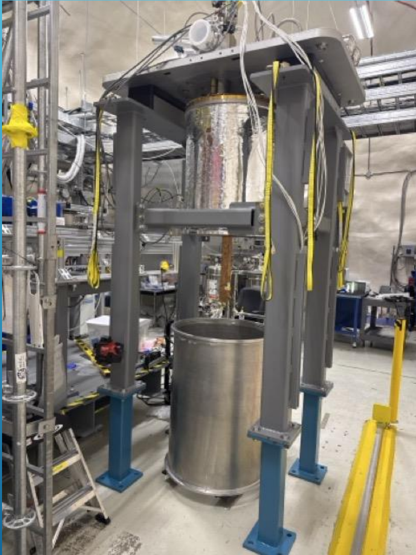
Dilution Fridge Tails installation
