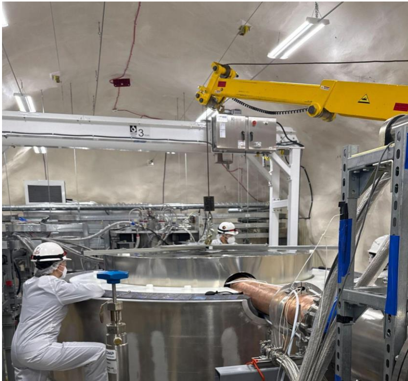
Installing top section of \mu -metal shield to protect detectors from Earth's magnetic field
