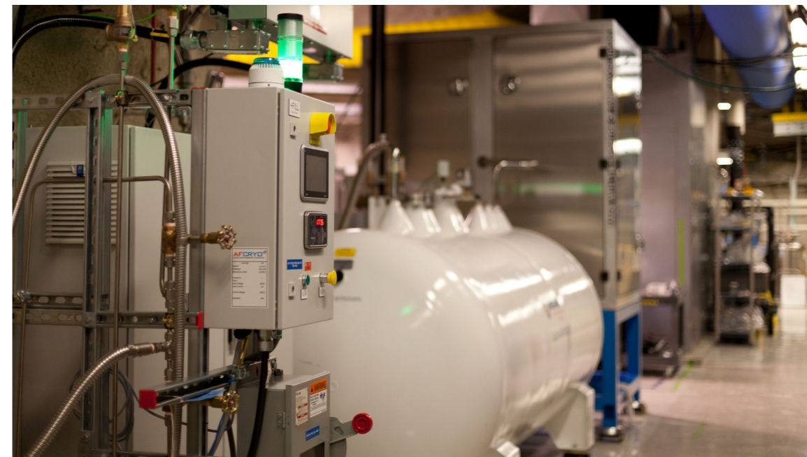
SNOLAB Liquid Nitrogen plant
